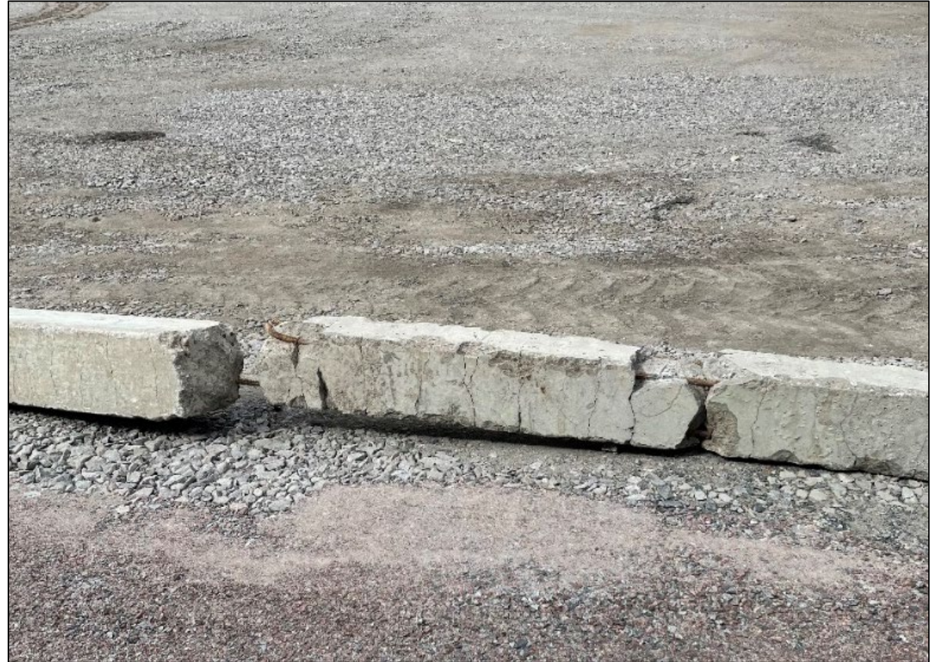
Reinforced concrete pile damaged due to hard driving conditions for a civil construction project in Sweden.
