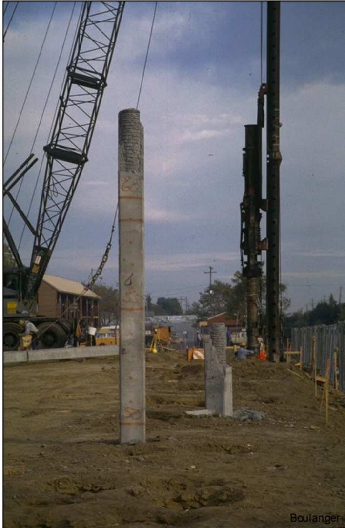
Reinforced concrete piles damaged during driving at a site in California | R. Boulanger (University of California)
