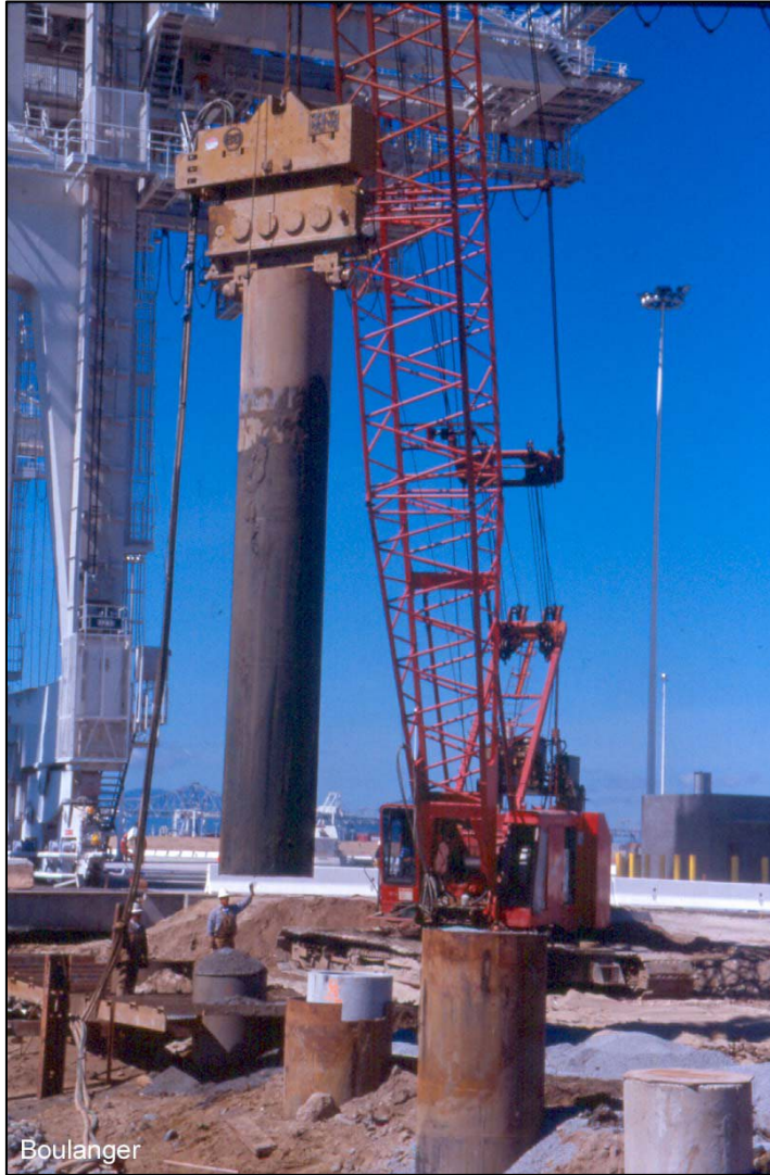
Steel pipe pile encountered an obstruction in the ground before its target elevation | R. Boulanger (University of California)
