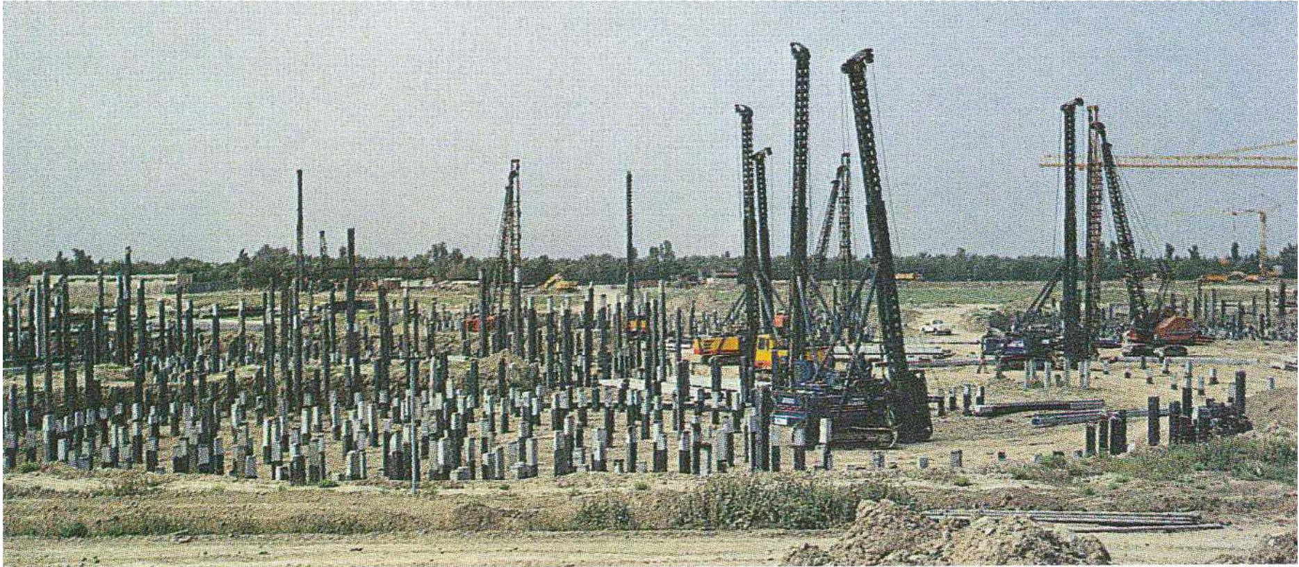
Piling for water treatment plant at Karkh Project Iraq, showing 6 BANUT rigs and 3 NCK rigs in operation.
